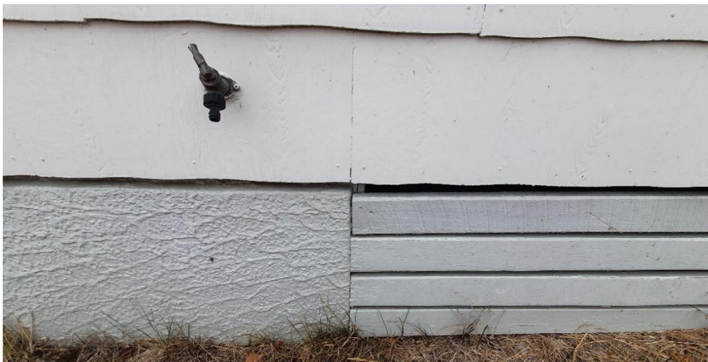
Photograph B5: Cladding and foundation detail including textured (stucco) render, painted timber and duroc cement sheet cladding.
