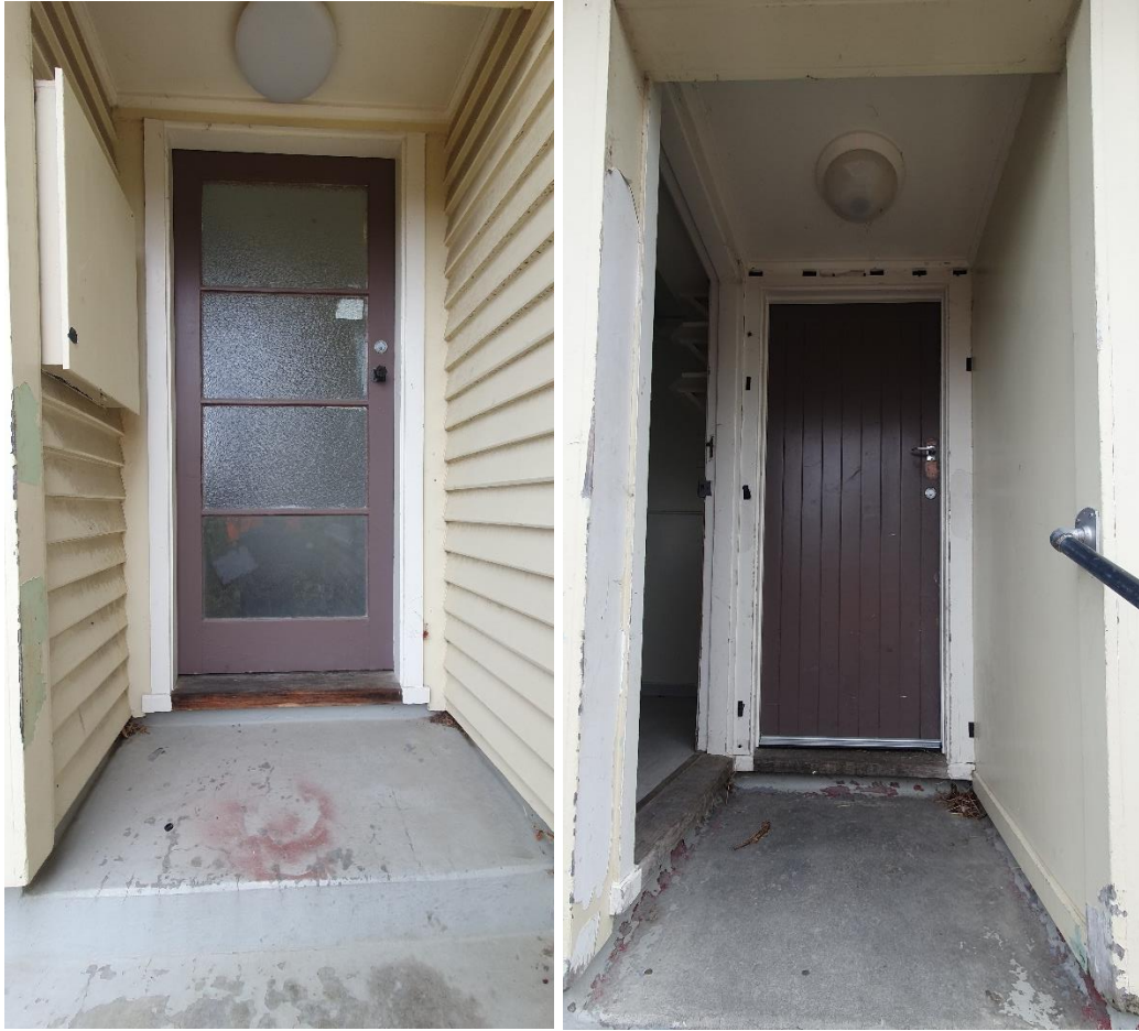
Photograph B17 (left) and B18 (right): Dwelling's front and side entryways, respectively; PACM ceiling and weatherboard walls at front entrance. PACM ceiling and walls at side entrance.
