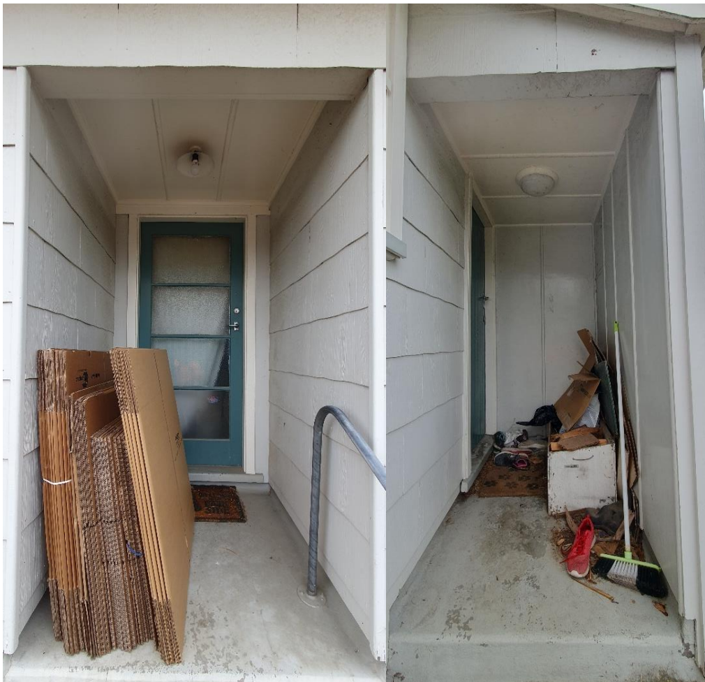
Photograph B7 (left) and B8 (right): Dwelling's front and rear entryways, respectively; PACM walls and ceiling at both.
