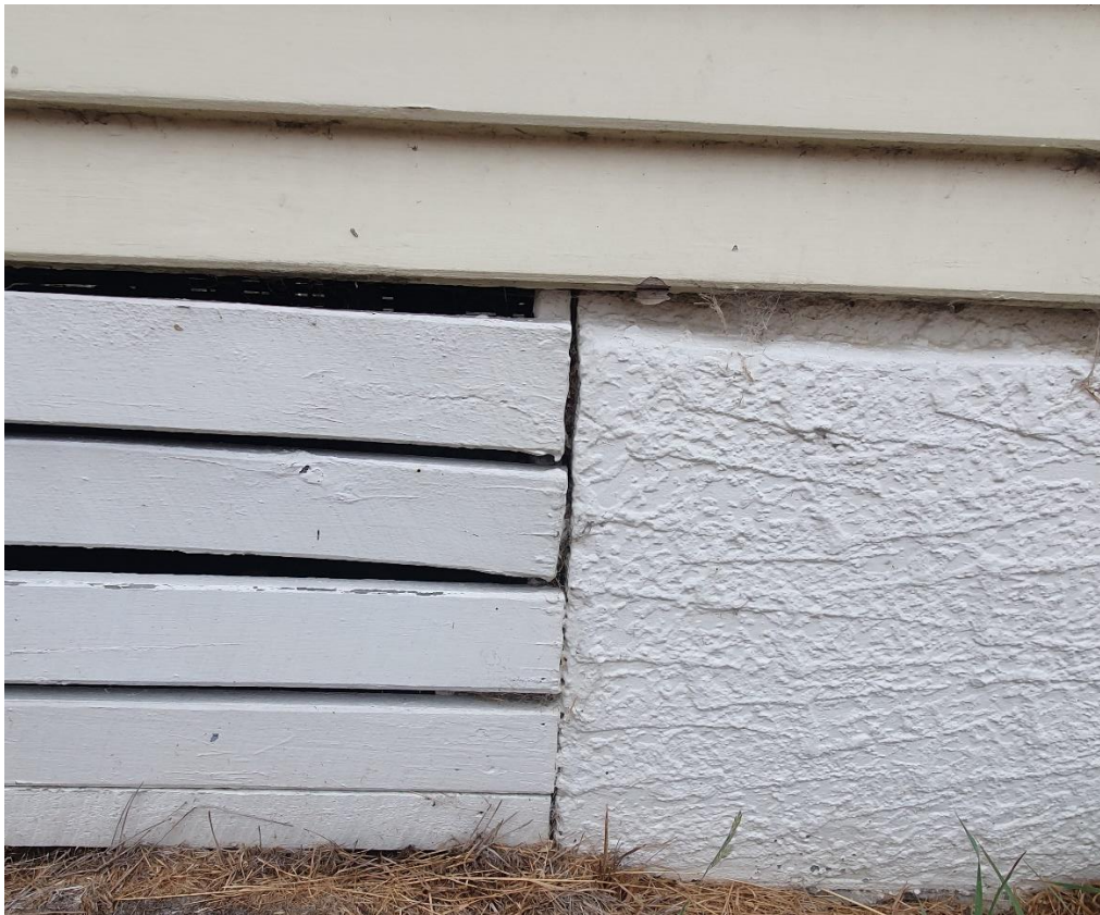
Photograph B16: Cladding and foundation detail including textured (stucco) render, painted timber, and weatherboard cladding.
