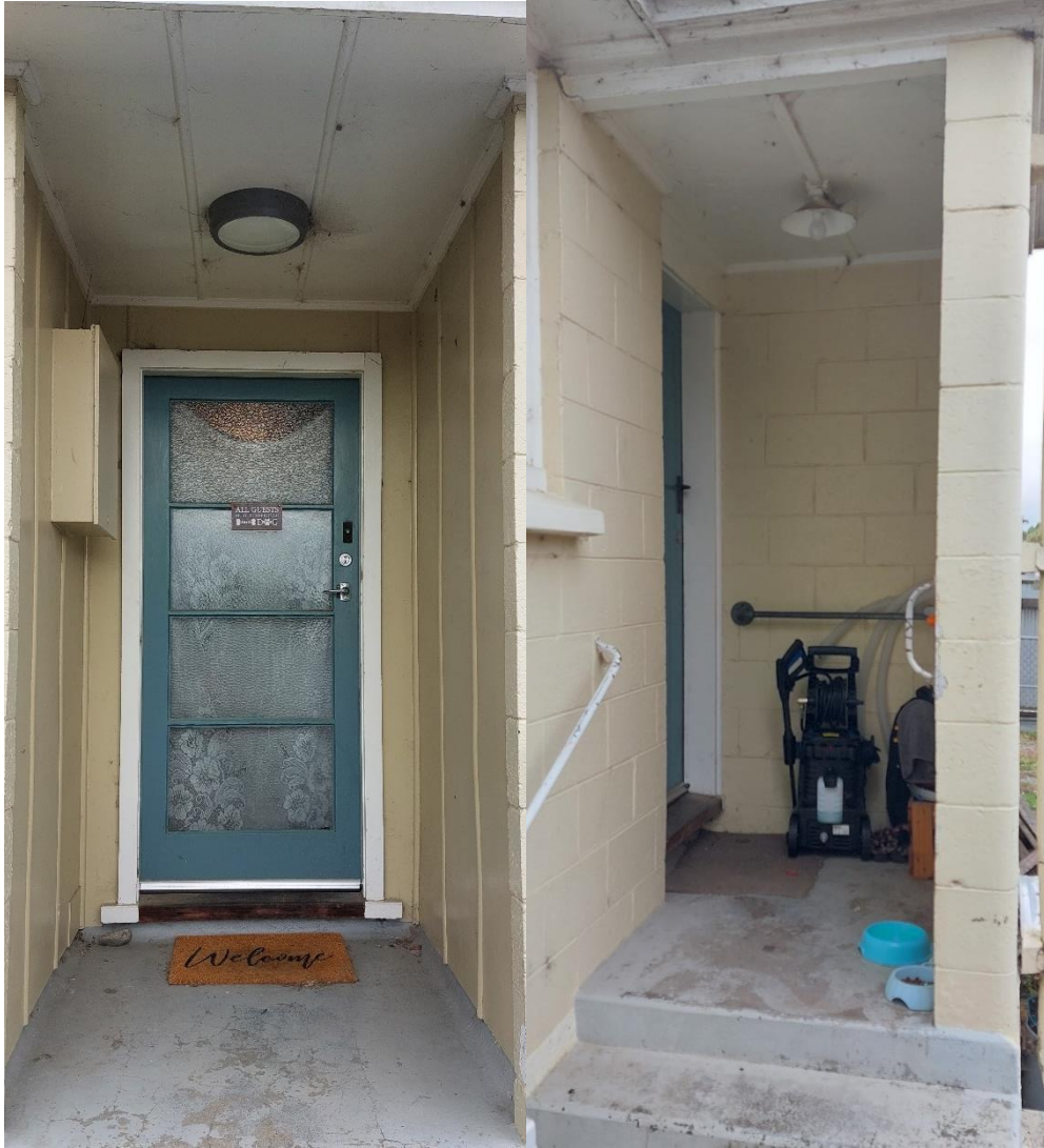
Photograph B25 (left) and B26 (right): Dwelling's front and rear entryways, respectively; PACM ceiling and walls at front entrance. PACM ceiling and painted concrete block walls at rear entrance.
