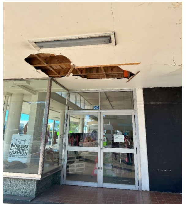
Main Street building decay. Gladstone Rd
