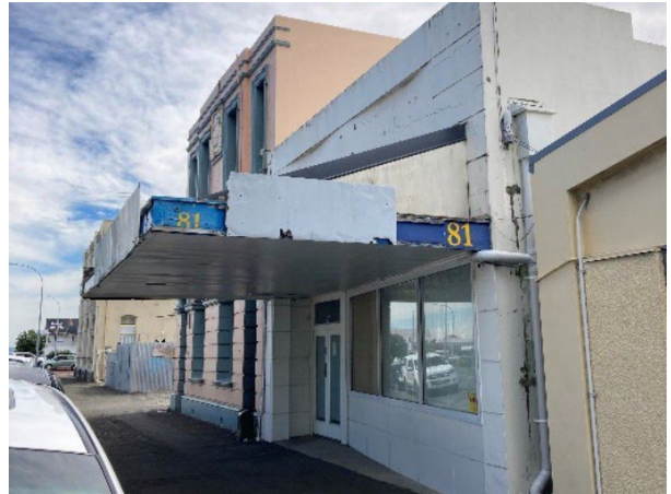
Deteriorating building. Childers Rd
