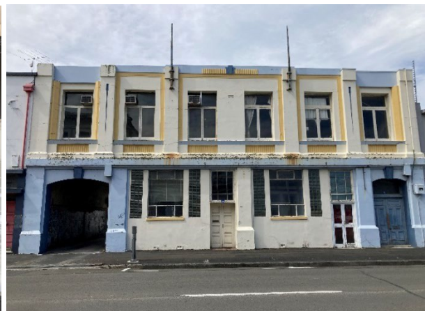
Deteriorating building. Lowe St
