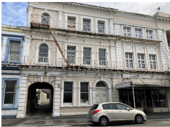
Masonic Hotel decaying façade. Lowe St
