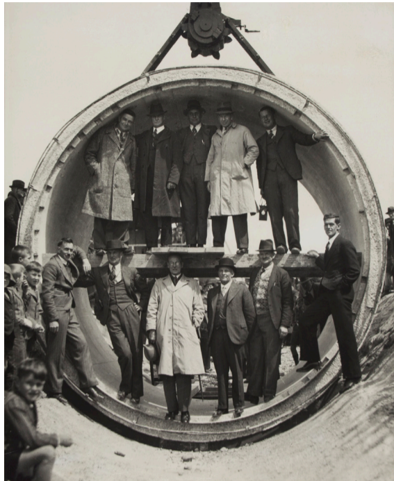
Left: The first pipe placed in the Rangitata Diversion Race at Surrey Hills in 1940. AM&HS collection, ref. 04.1997.0146
