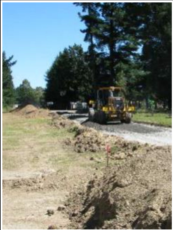
Chertsey WTP UV/Filtration Upgrade
