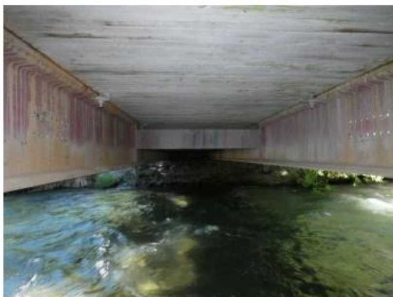
(a) Corrosion of steel members
