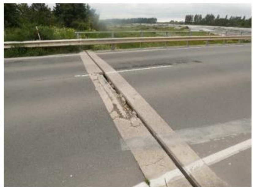
(b) Failed expansion joint
