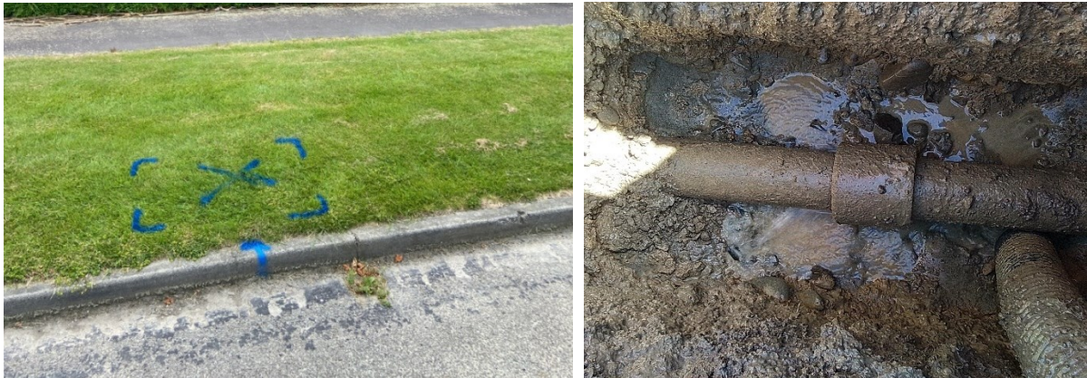
Figure 9 - 35L/minute leak. Surface view and actual fault (leaking joint)
