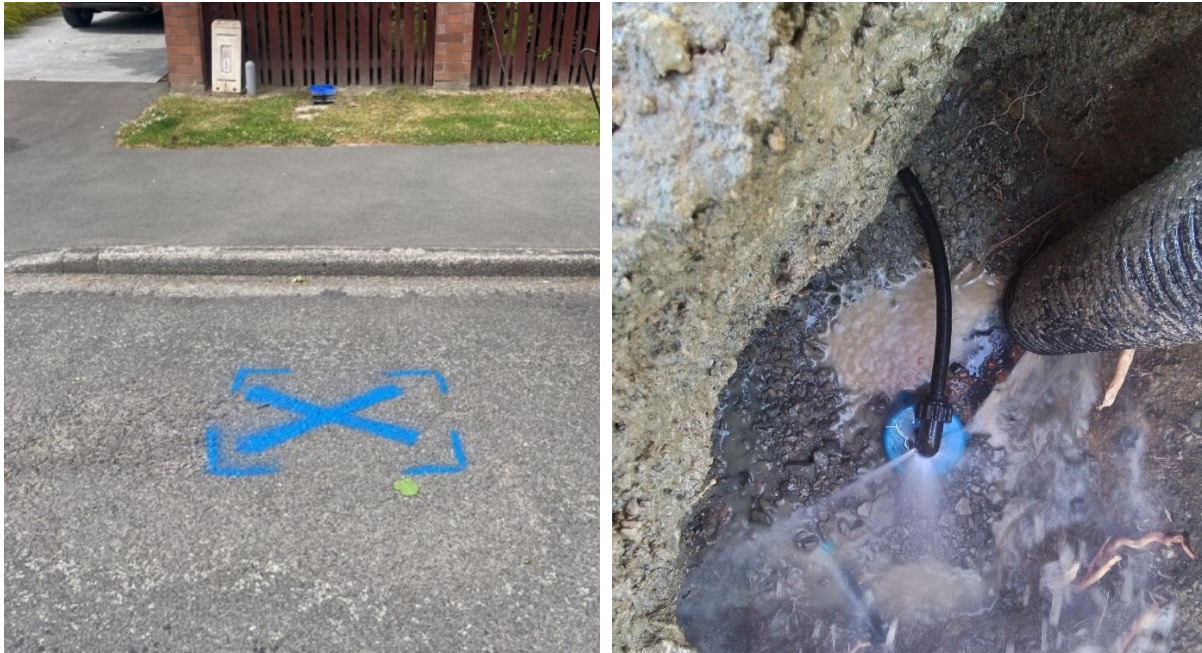
Figure 10 - 15L/minute leak. Surface view and actual fault (leaking fitting)
