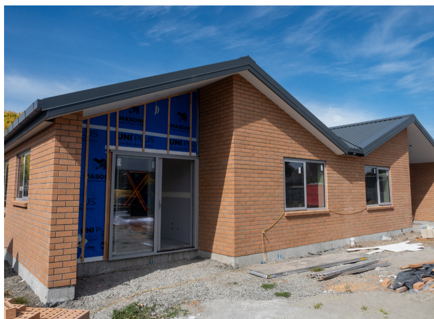
FRIENDSHIP LANE SHAPING UP: Bricks are currently being installed on the 16 new Elderly Persons Housing units, as the project tracks on schedule toward a mid-year completion. Drainlayers are also on site working on drains, stormwater and sewer. Interior painting is expected to begin later this month.
