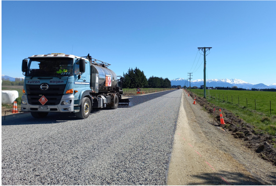
The first rehabilitated section of Ashburton Staveley Road has been sealed, ahead of schedule thanks to fine weather.
