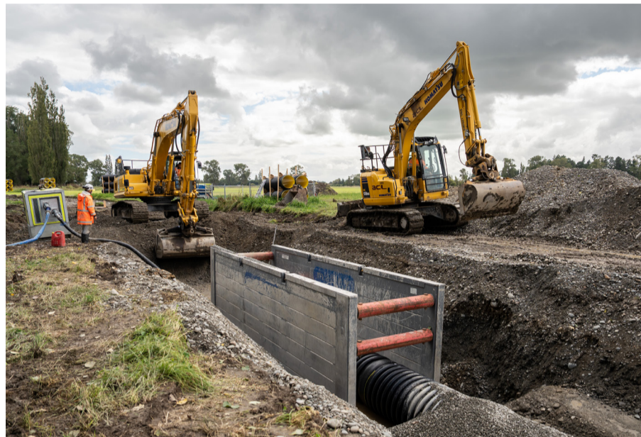
Contractors at work installing a new sewer main between Trevors Road and Milton Road, to transfer Ashburton wastewater to the Wilkins Road treatment plant.
